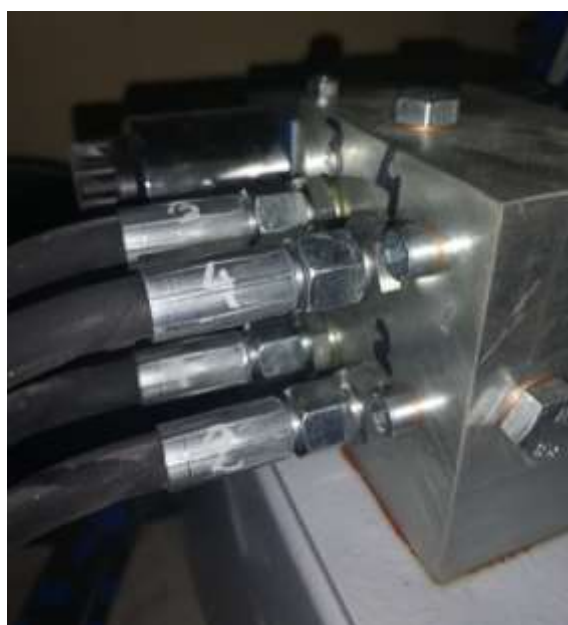
Fig. 19 - Hydraulic power supply cube with connected hydraulic hoses
