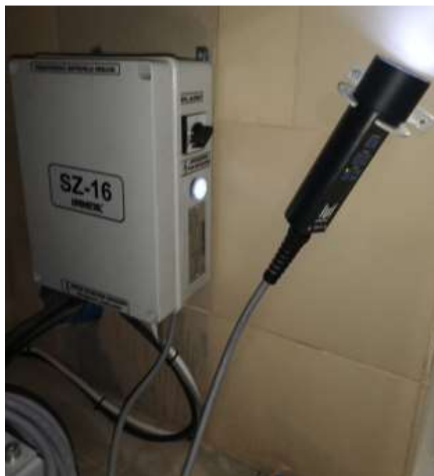
Fig. 20 - Electrical box and torch holder with torch mounted in the diagnostic pit recess
